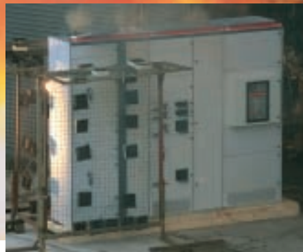
Low voltage switchgear during test
